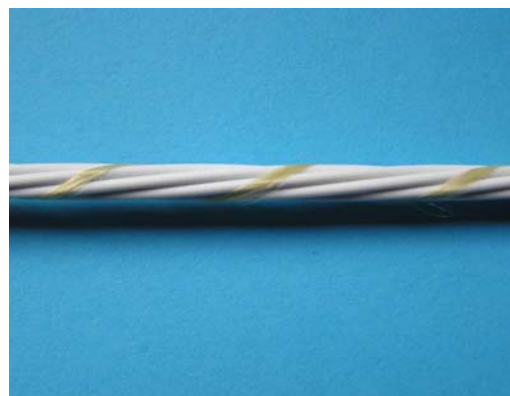
NOT ACCEPTABLE Binder wrapped in wrong direction
