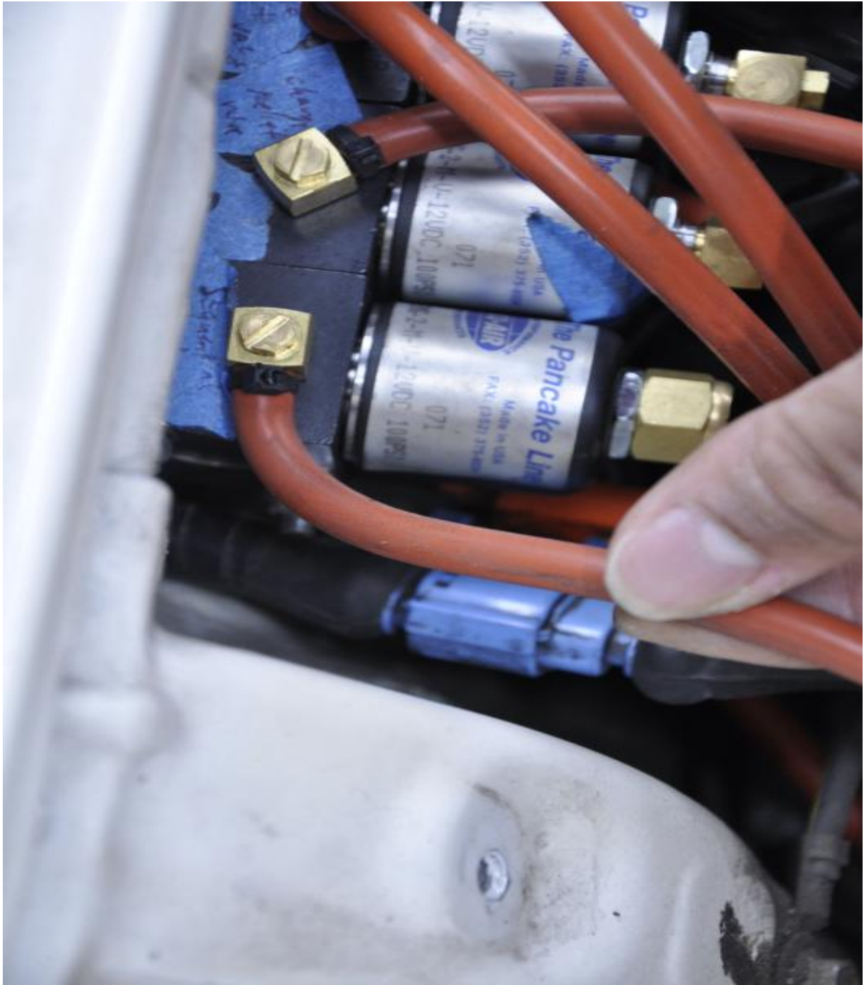
Refer to DARK BLUE routing on vacuum diagram, connect from port B of solenoid E
