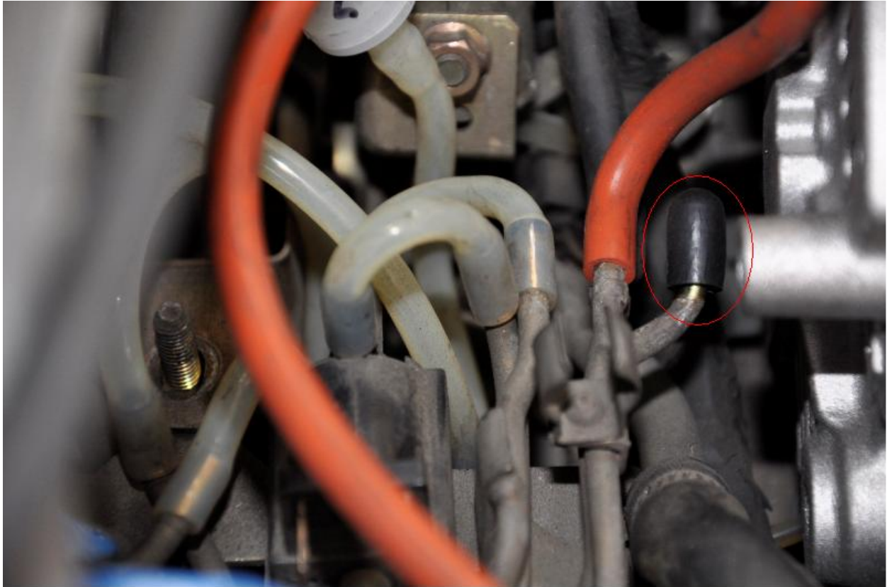
This picture showed the vacuum lines from previous picture in close-up, cap this open metal vacuum line on the right.
